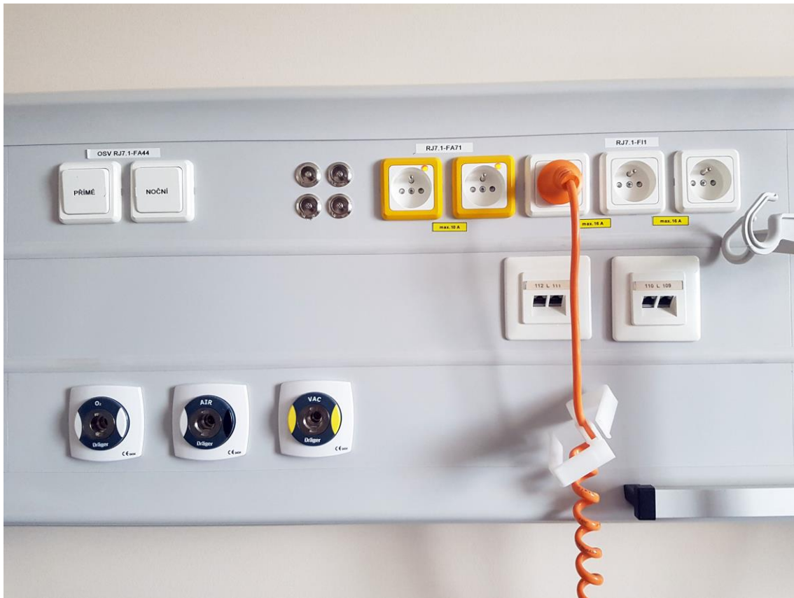
Medical Gas and Electric Headwalls wall-mounted
