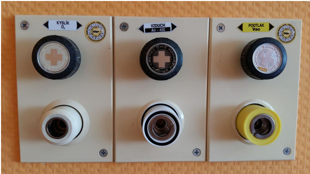
Central gas distribution
