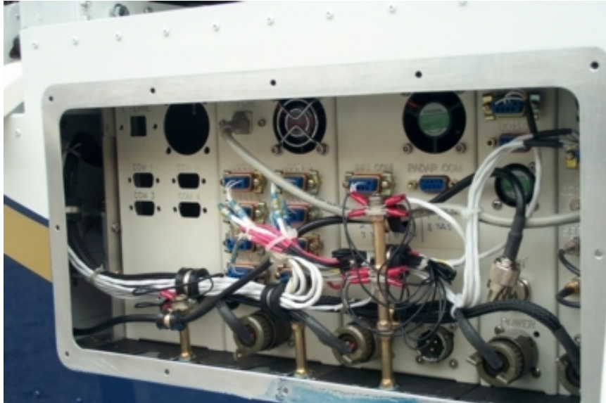
Figure 7: Module back panels with wiring harness
