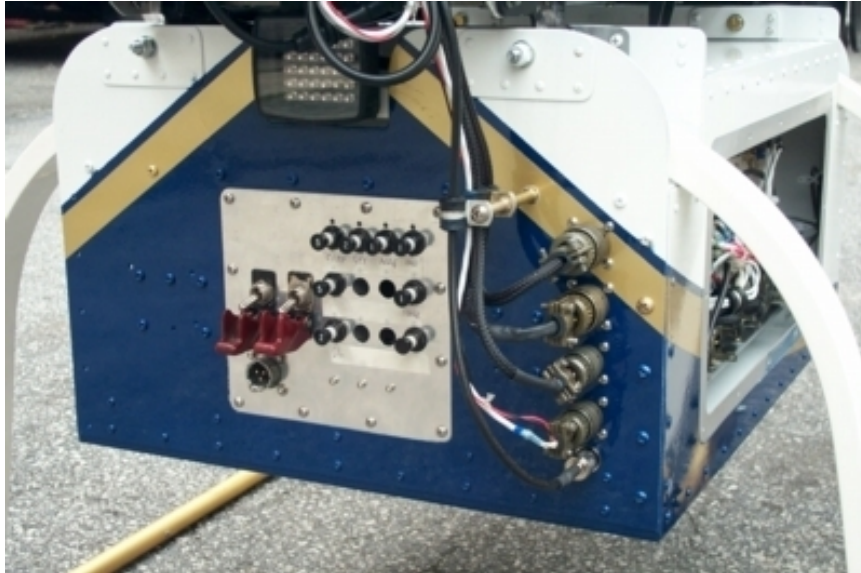
Figure 9: Power panel on the back of the avionics box
