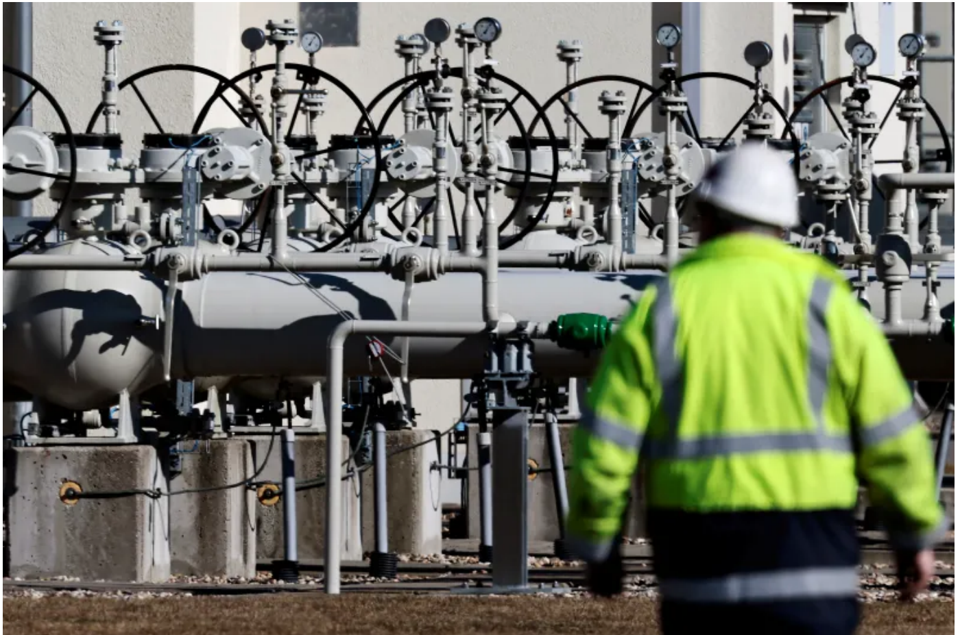
Gas pipeline equipment in Lubmin, Germany, March 2022
