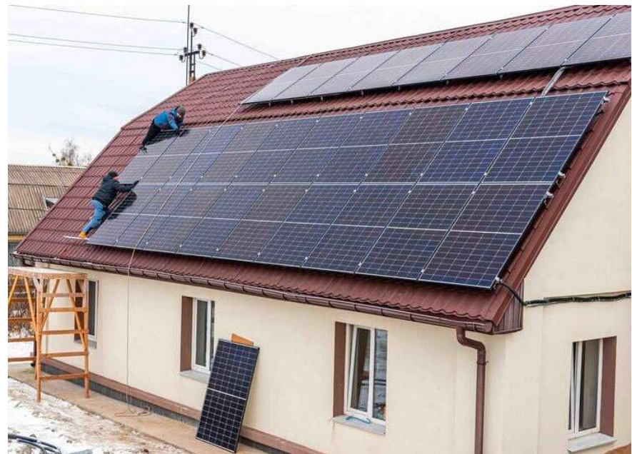
Solar panels on the roof of Horenka hospital. Source: Greenpeace
