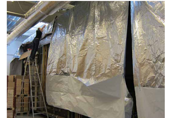
Fig. 32: View of the painting storage 1 at the old Inzersdorf facility shortly before the beginning of anoxic nitrogen treatment. The left hand side of the picture shows how the special foil, which at the back and sides has already been heat-sealed and adhered to the floor, is now being closed at the front as well for anoxic nitrogen treatment.
