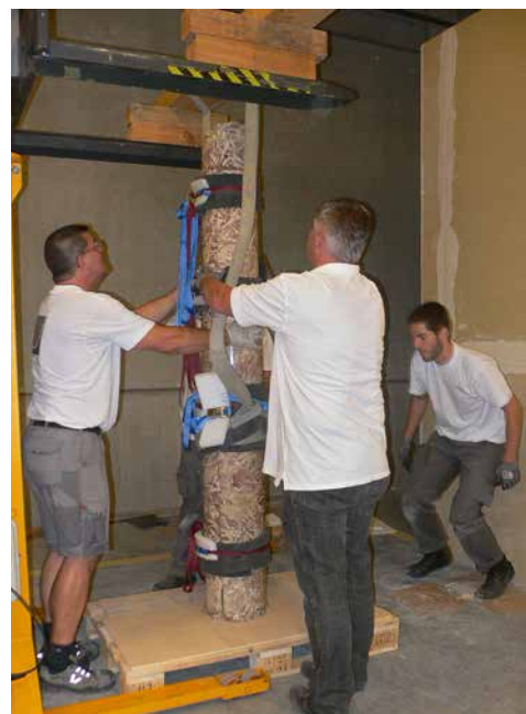
Fig. 57: Raising a stabilised stone column with a continuous crack formation with the help of a lifting device.
