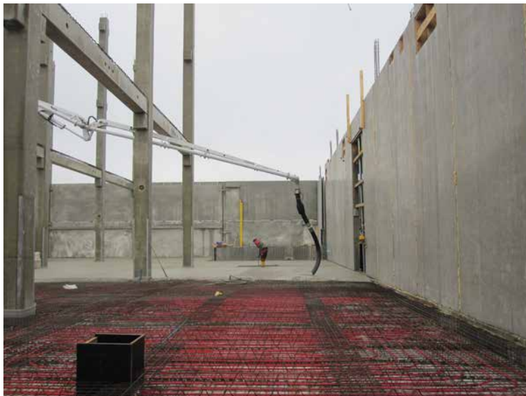
Fig. 4: Addition of concrete to the ceilings with concrete core activation and reinforcement already in place.
