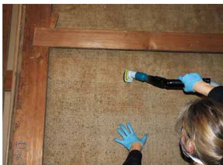
Fig. 12: Old, inactive mould spores were cleaned away using vacuum cleaners equipped with HEPA-filters.
