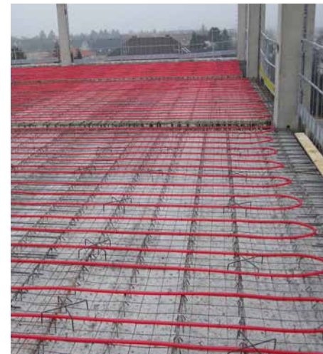
Fig. 5: The activated floors provide a stable climate. The photograph shows the installation of the tubing for the concrete core activation before the concrete has been poured.
