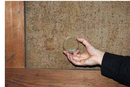
Fig. 6: Sampling of a painting contaminated with mould.
