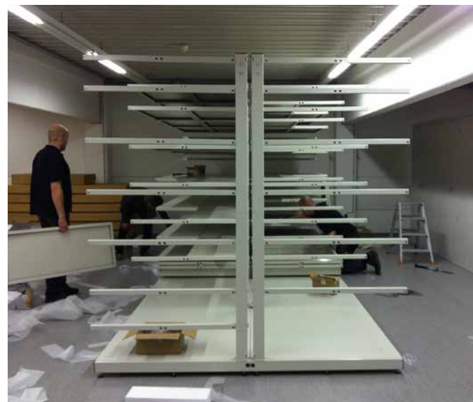
Fig. 35: Assembly of the prototype for the support-free shelving at the storage facility Inzersdorf.
