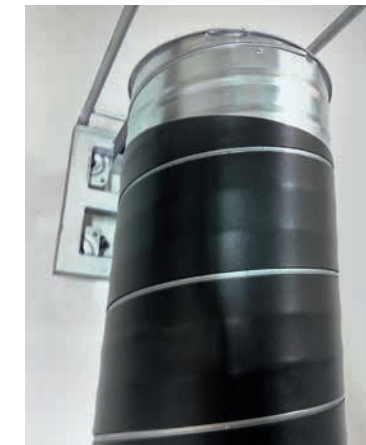
Fig. 6: Wrapping of the folded spiral-seam pipes with Plastazote (PE foam) cut into narrow strips (first step).
