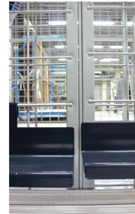
Fig. 4: The installation should be monitored very closely. At the new storage facility, the fact that the wire mesh panels had not been assembled so that they fit perfectly in some places was only noticed relatively late. The resulting slight misalignment is especially bothersome when using the additional support elements to be hooked in individually. Unfortunately this could not be rectified, as a very large number of paintings had already been hung on the racks at that point.
