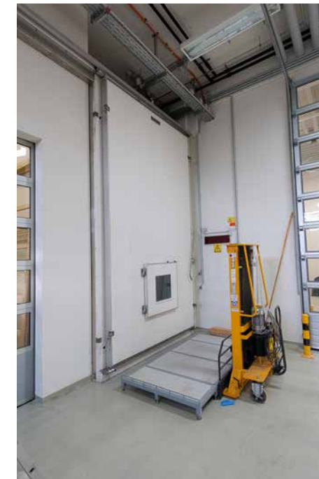
Fig. 69: Anoxic nitrogen treatment chamber in the central art storage facility of the Kunsthistorisches Museum Vienna.
