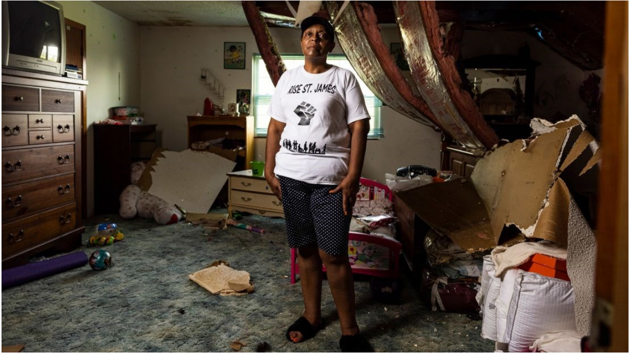
Sharon Lavigne's home was heavily damaged by Hurricane Ida. Edmund D. Fountain for CNN
