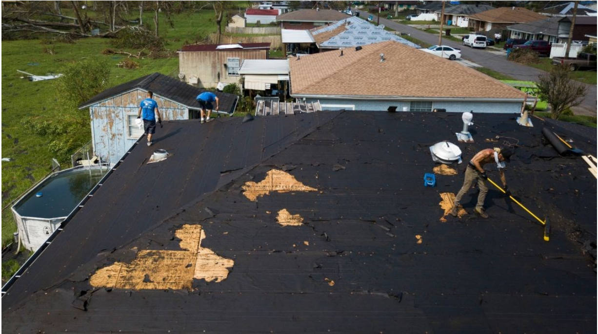
People work to repair a roof in Norco, Louisiana. Edmund D. Fountain for CNN
