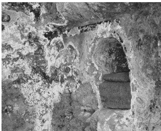
FIGURE 5.5 Salting on the internal walls of the tomb of Servilia, Carmona, Spain.
