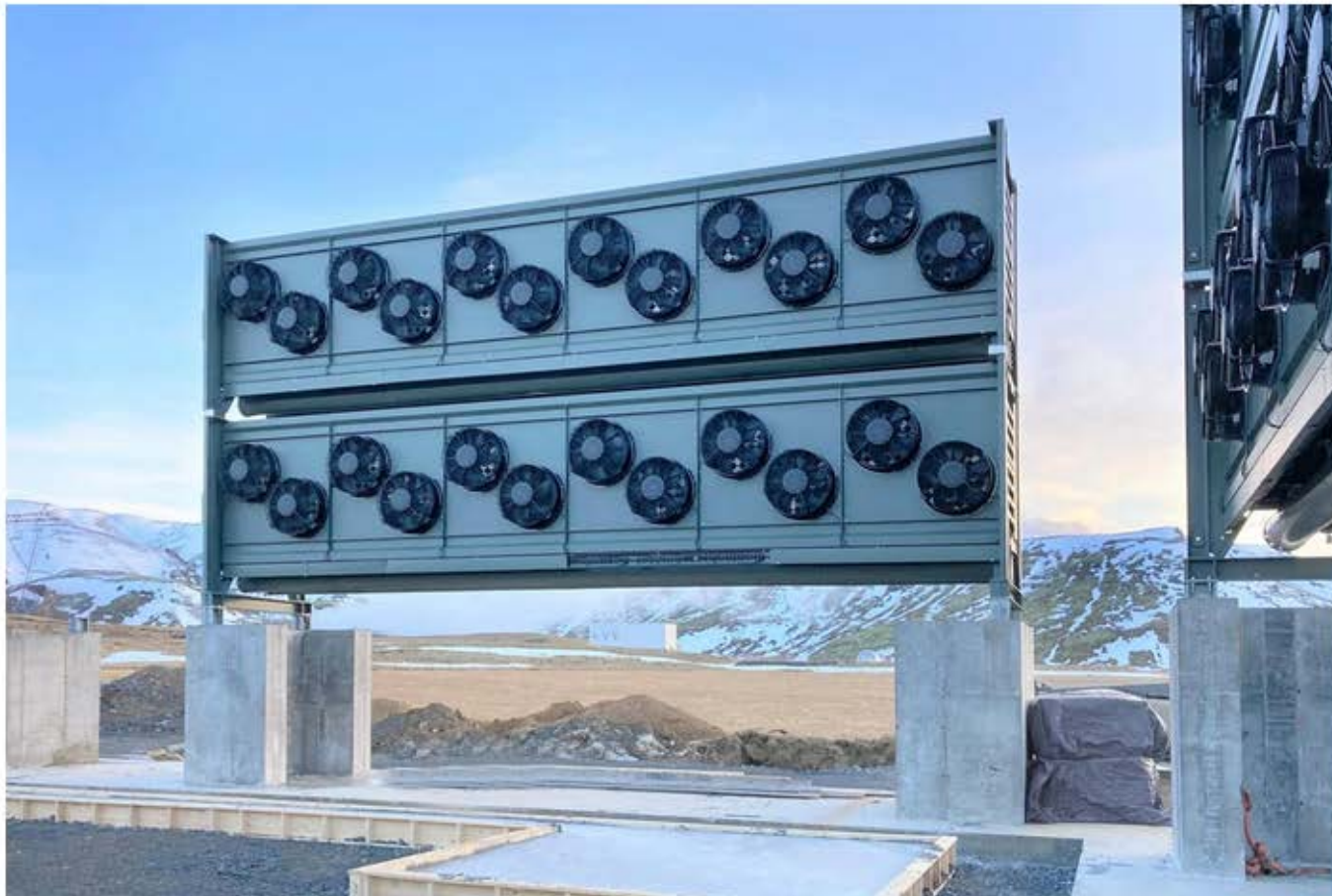
▲ The Orca plant in Climevents, Iceland, intends to extract 4,000 tonnes of CO2 per year from the air. Climevents
