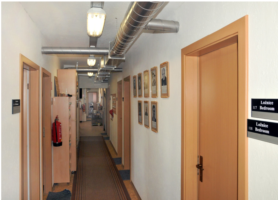
Fig. 11. Central line (along the corridor) and lateral branches of pipes that form a part of heating system delivering hot air to individual rooms. © Photo: K. Láška.
