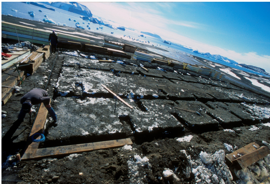
Fig. 3. Foundations of main building create the graps made from oak railway sleepers. © Photo: H. Adámek.
