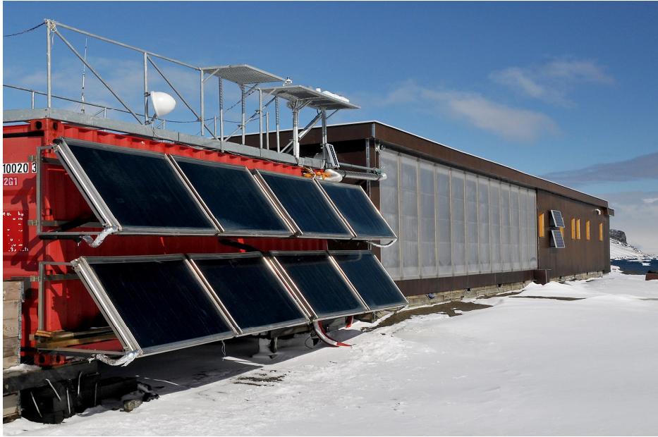
Fig. 10. Hot air collectors (total surface 36 \text{ m}^2 ) on the north side of main building (right side) and thermal panels (total surface 12 \text{ m}^2 ) installed on the wall of incinerator container (left side). © Photo: K. Láška.
