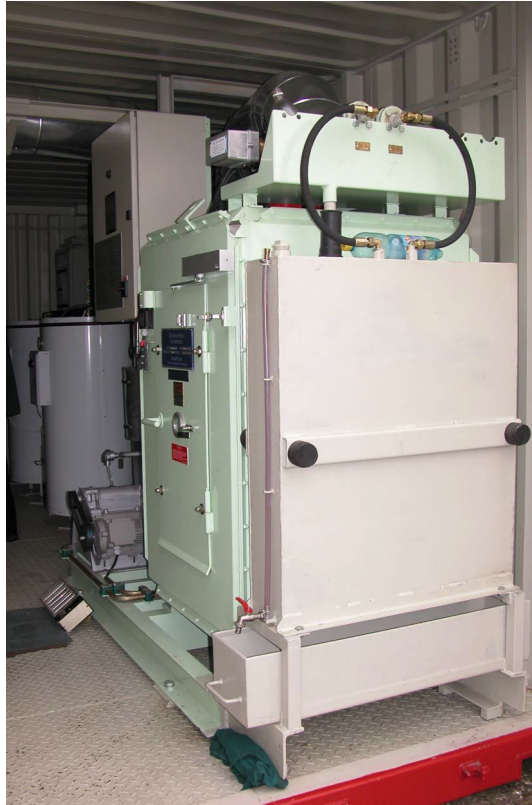
Fig. 17. An OG120SW marine incinerator, right: part of engine room of power supply generators. © Photo: P. Prošek.
