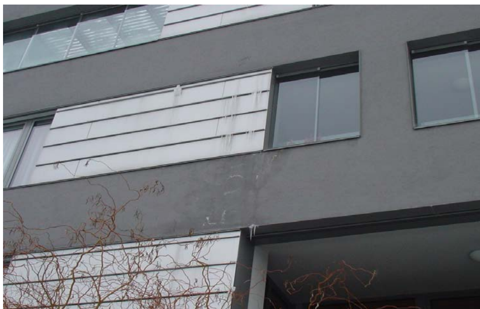
Obr. 3 – Defekt alukobundu v zimě - rampouchy Fig. 3 – Alukobond defect in winter - icicles
