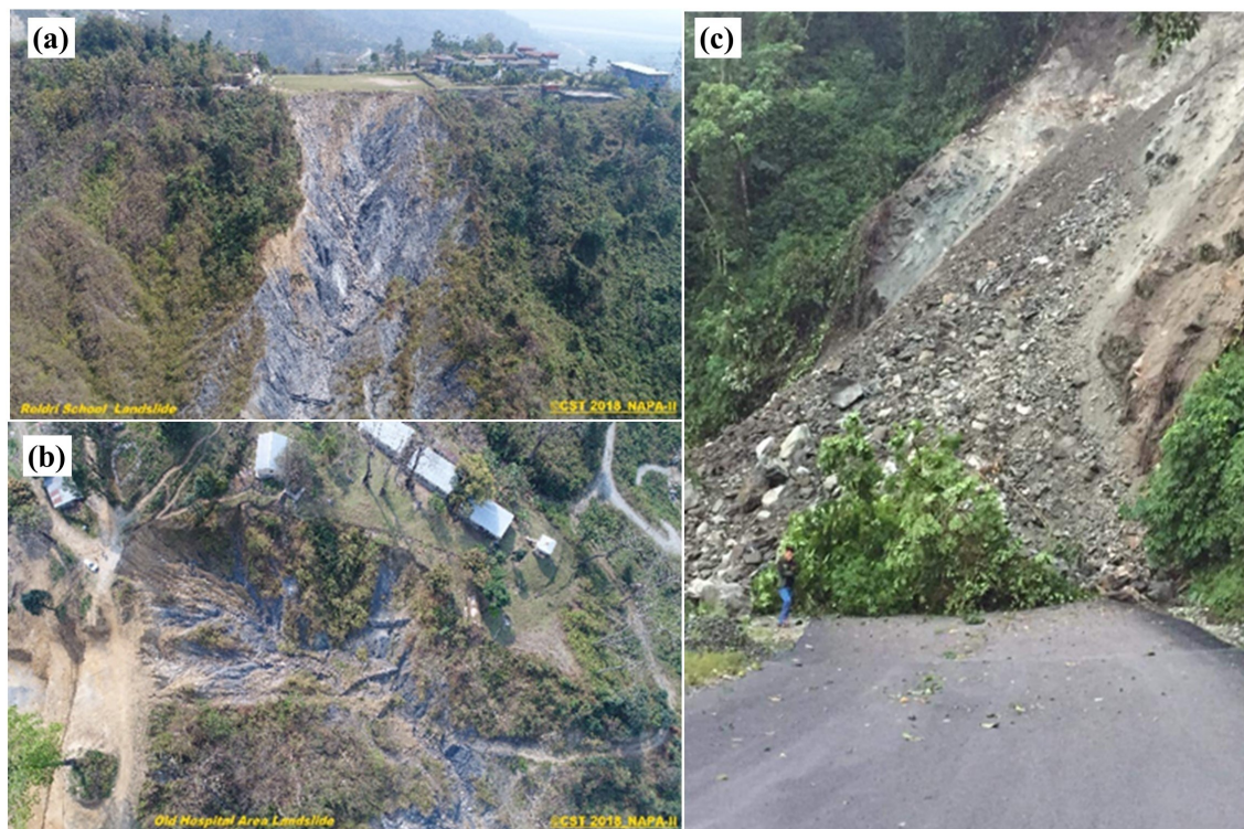
Figure 2. (a,b) Road and infrastructure affected by landslide at 5 km chainage, Rinchening and (c) Landslides roadblock at 17 km chainage, Sorchen, in the study area (photo courtesy: College of Science and Technology).
