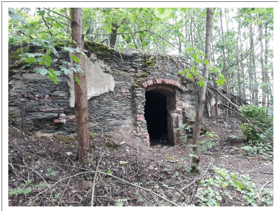
Picture 6. The dilapidated pilgrim Church of St. Anne in its current state.
