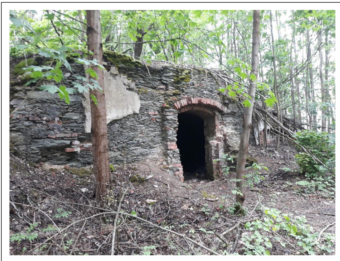
Picture 6. The dilapidated pilgrim Church of St. Anne in its current state.
